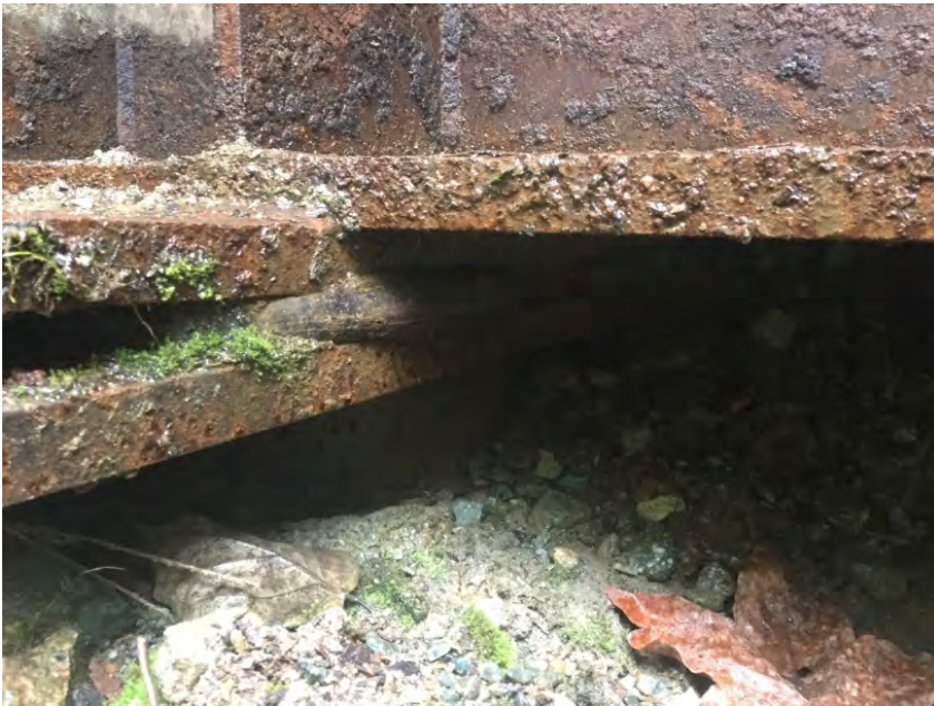
Bulging bearing pads at left bank
