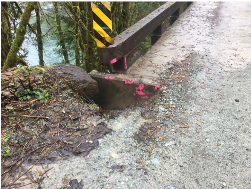
Eroding fill at DS left approach from surface runoff
